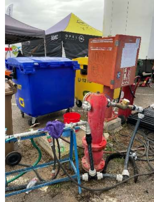
Access to hydrant and emergency services is blocked
