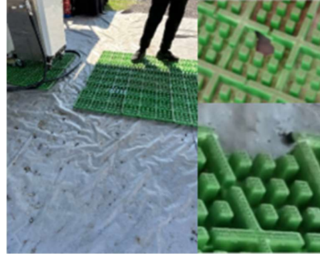
Broken mats at Refueling increase the chance of ground pollution in case of spillage
